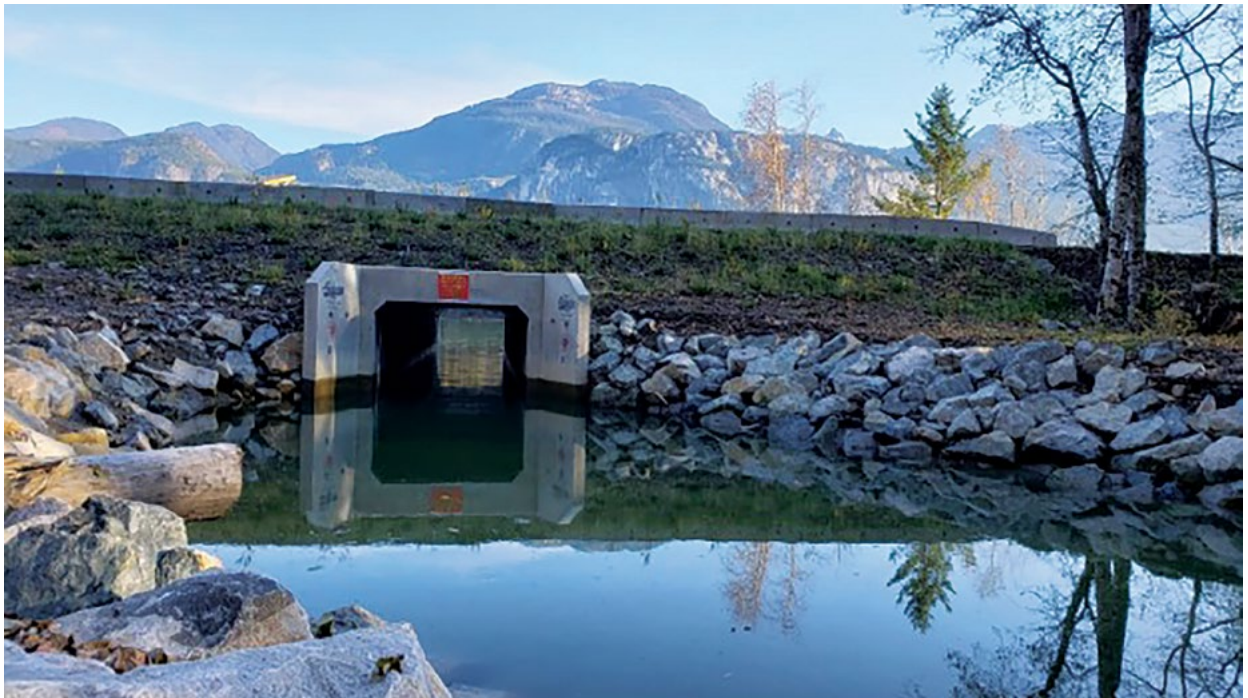
A box culvert installed in the dike to increase connectivity between the Squamish River and the estuary. (Credit: Edith Tobe)
