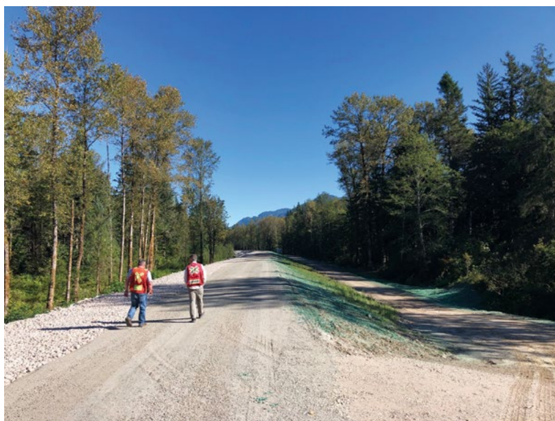
A view along the Squamish River dike upgrade, undertaken in 2019. (Credit: David Roulston)
